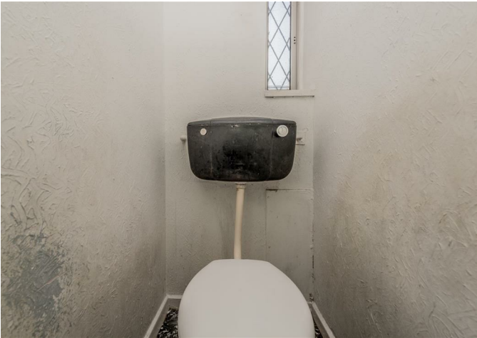
Double glazed window, low flush WC
