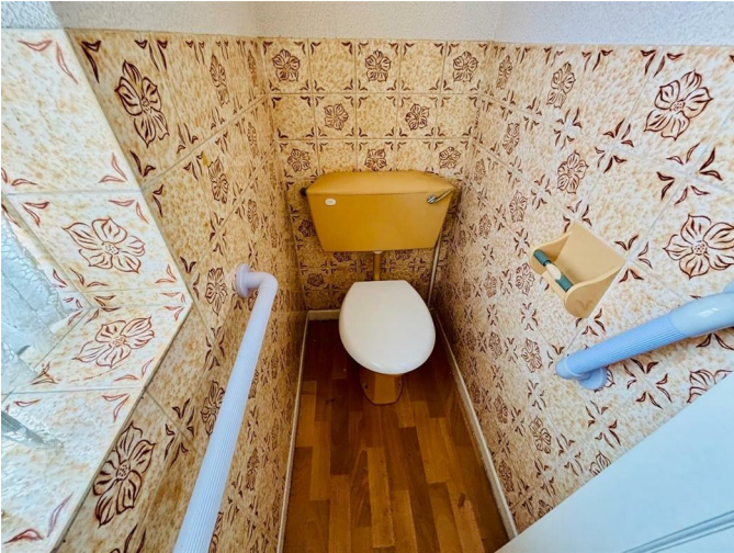
Double glazed window, low flush WC
