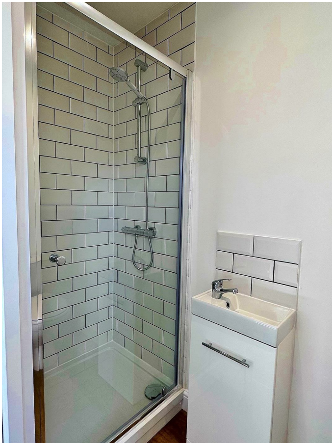
Tiled shower cubicle with wall mounted shower unit and glazed screen. Low level WC. Wash basin with cupboard below. Inset ceiling spotlights.
