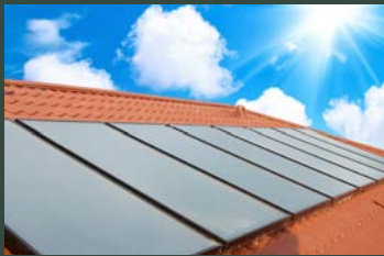
Solar PV panels
