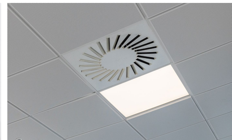
AIR CONDITIONING | RAISED FLOORS
