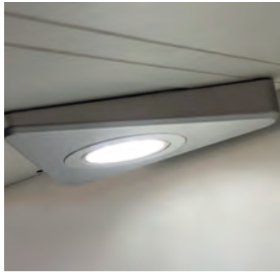
Low energy lighting throughout with LED downlights to kitchen, hallway, Cloakroom and bathrooms
