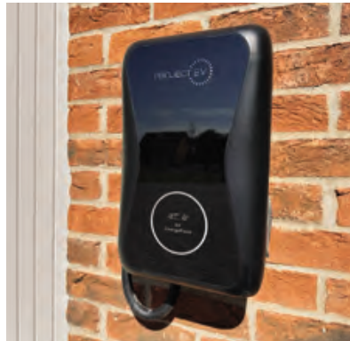
Electric car charging point
