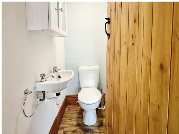
Low level WC, wash hand basin.
