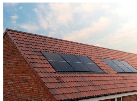
PV solar panels fitted to every home contributing to the low running costs of all Hartfell homes
