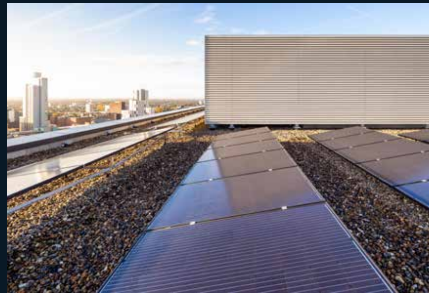
Landmark rooftop solar panels
