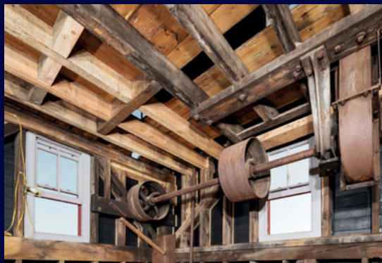
Hoist machinery in the Jubilee Tower © Historic England
