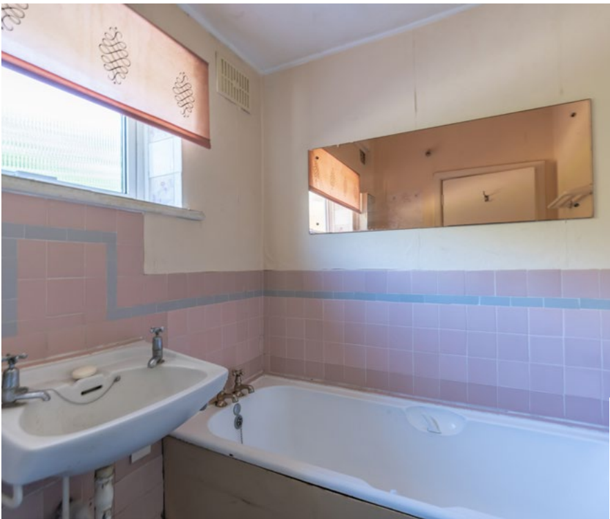
It is in need of complete modernisation throughout.
