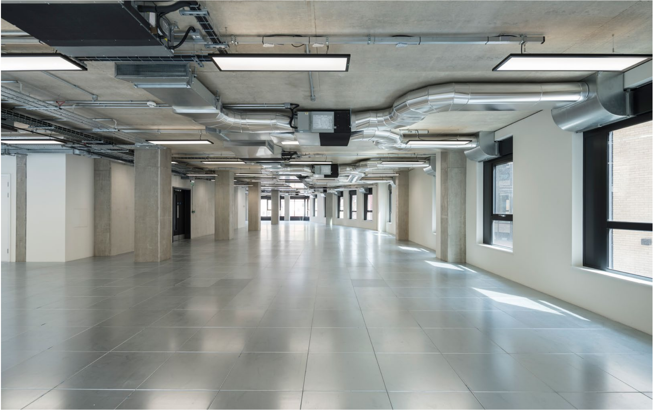
No.1 The Distillery – Typical upper floor, excellent natural light and fantastic views
