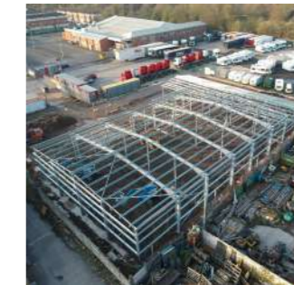
Phase I steel portal frame with a similar design strategy to be adopted in Phase II. The supply chain from Phase I is to be generally retained on Phase II
