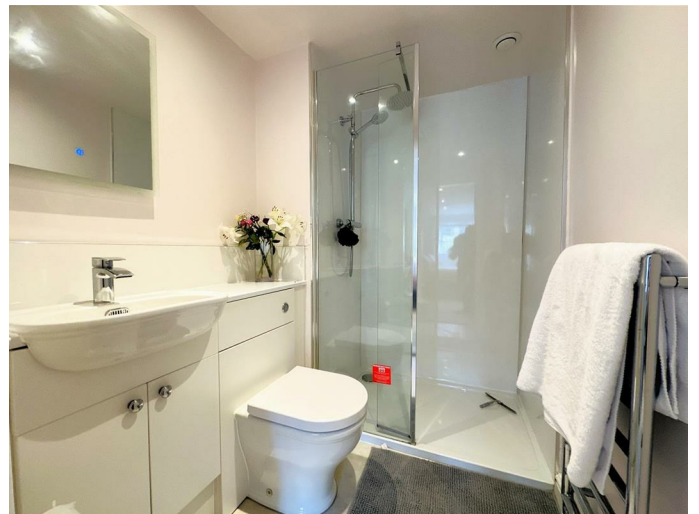
Walk in shower cubicle with fixed head shower over with further attachment. The area is wet walled to ceiling height. White low flush w.c with hidden cistern, chrome controls and white wash hand basin with chrome mixer tap over; both set into white vanity unit with chrome handles and splashback. Chrome heated towel rail and extractor fan.
