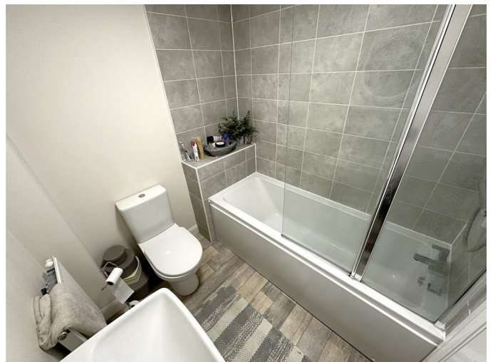
Toilet, wash hand basin, bath with mains shower over, extractor fan and part tiled.
