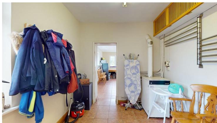
Trianco oil fired boiler providing heating and hot water, double glazed window, terracotta style ceramic tile flooring.
