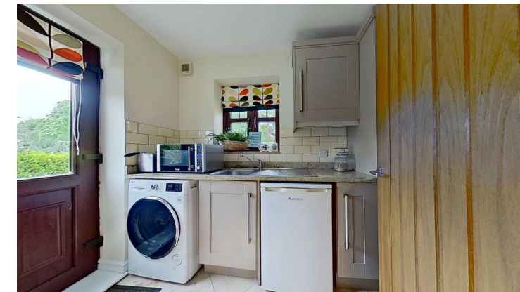
Fitted base units with granite worktop and matching upstands. Inset single bowl stainless steel sink unit and drainer with chrome mixer. Tall cupboard housing a Glow Worm 18SX1 condensing gas fired central heating boiler, plumbing and space for washing machine, space for freezer or tumble dryer, burglar alarm control pad, single radiator with thermostat, tiled splashback, travertine tiled floor, ceiling light point, extractor, UPVC double glazed window, and UPVC double glazed door to outside.
