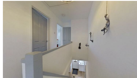
Ceiling light point, mains connected smoke alarm, and access to loft space. Doors to bedroom one, bedroom two, bedroom three and bathroom.
