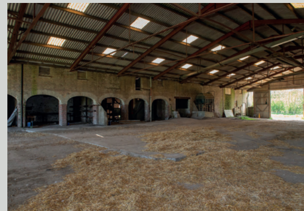
General purpose portal frame building (Building 15) (estimated GIA 1030.56 m 2 ) measuring internally 45.20 m x 22.80 m.
