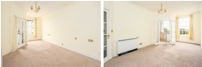
Electric storage heater Telephone point TV point Sash window to front elevation
