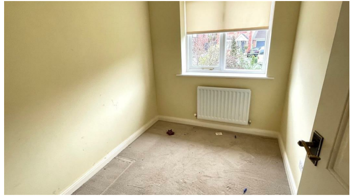
Double glazed window, radiator.
