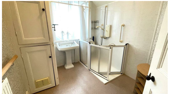
With walk in disability shower area with 'Mira advance' electric shower, plastic wall cladding, pedestal wash hand basin, extractor fan, non slip flooring, airing cupboard housing washing machine, 'Ideal Logic' combination central heating and hot water boiler, upvc double glazed window, radiator.
