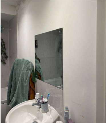
22-11-2024 10:58 / Bathroom Walls Ceilings / G9bm1mndp
