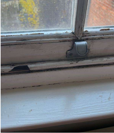
22-11-2024 10:59 / Bedroom Windows Sills / 0xdnb9cya
