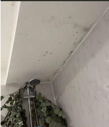
22-11-2024 10:58 / Bathroom Walls Ceilings / X4goq8itd
