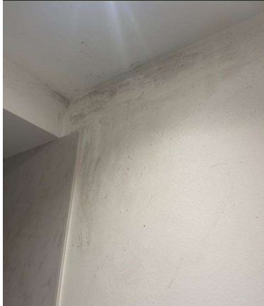
22-11-2024 10:58 / Bathroom Walls Ceilings / Zhcrfs6zd
